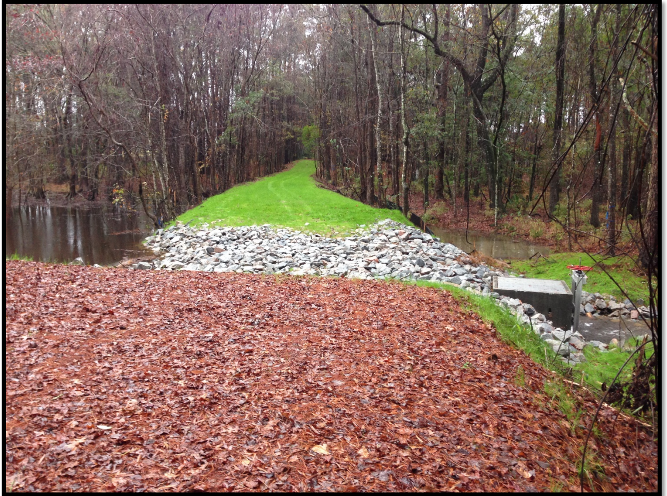
Figure 5-3 – Okatie East Wetland Enhancement Outlet Structure and Wetland Enhancement
